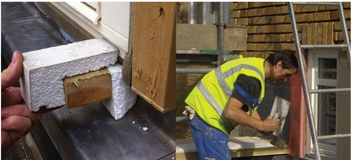
Application of EPS external wall insulation with brick slips on EnerPHit project by Grosvenor Britain and Ireland
